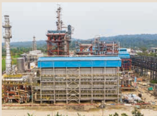
500 TPD Methanol Plant
