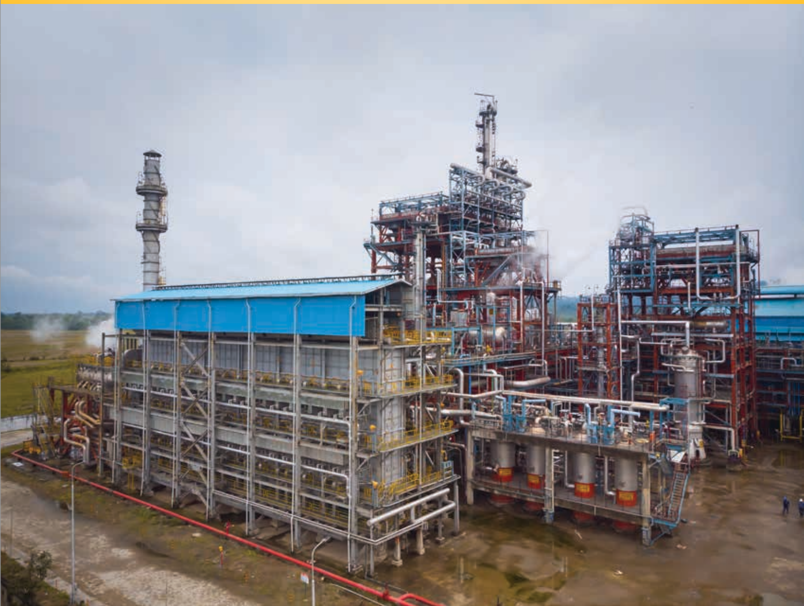
500 TPD Methanol Plant
